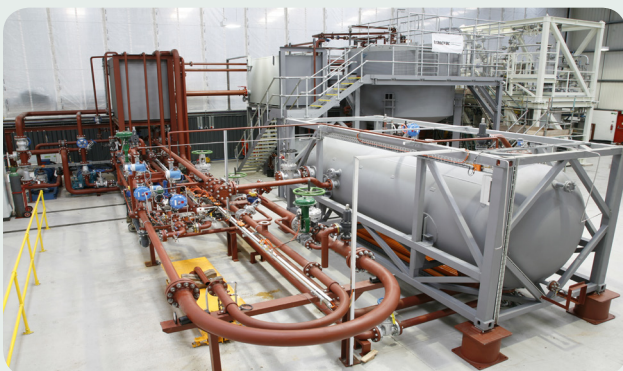
Transvac's new R&D Facility - Capable of pressures up to 120barg, Flows up to 700m 3 /hr
